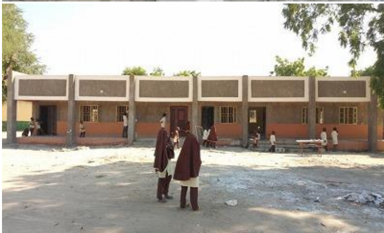
During and After rehabilitation of one of classroom buildings of Mafa Primary School
